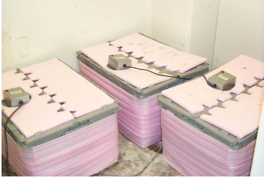
Figure 2 – Hot Water Tanks with Water Temperature Controls
