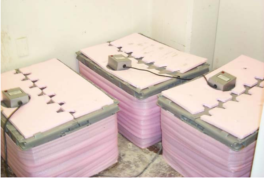
Figure 2 – Hot Water Tanks with Water Temperature Controls
