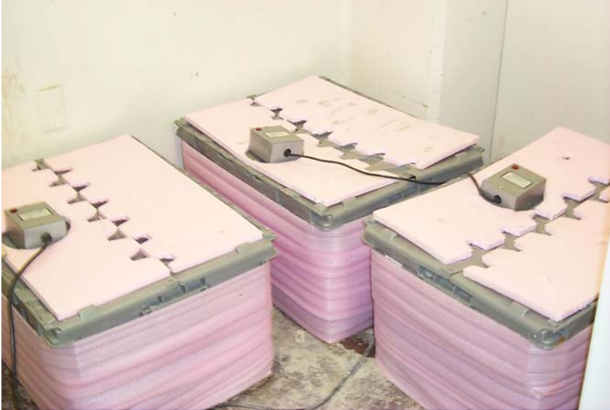
Figure 2 – Hot Water Tanks with Water Temperature Controls
